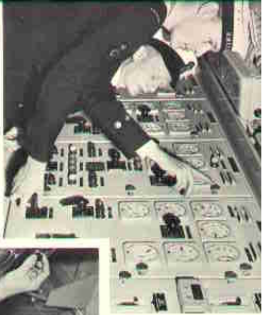
The main switchboard
