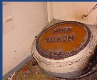
Welded plate over starboard side of aluminum hoist
